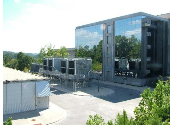
AT&T Regional Data Center
