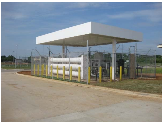
CNG Facility - Athens, AL 1
